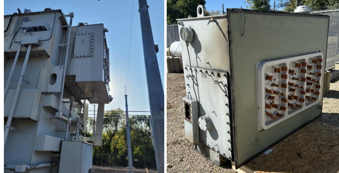
Before LTC Replacement
