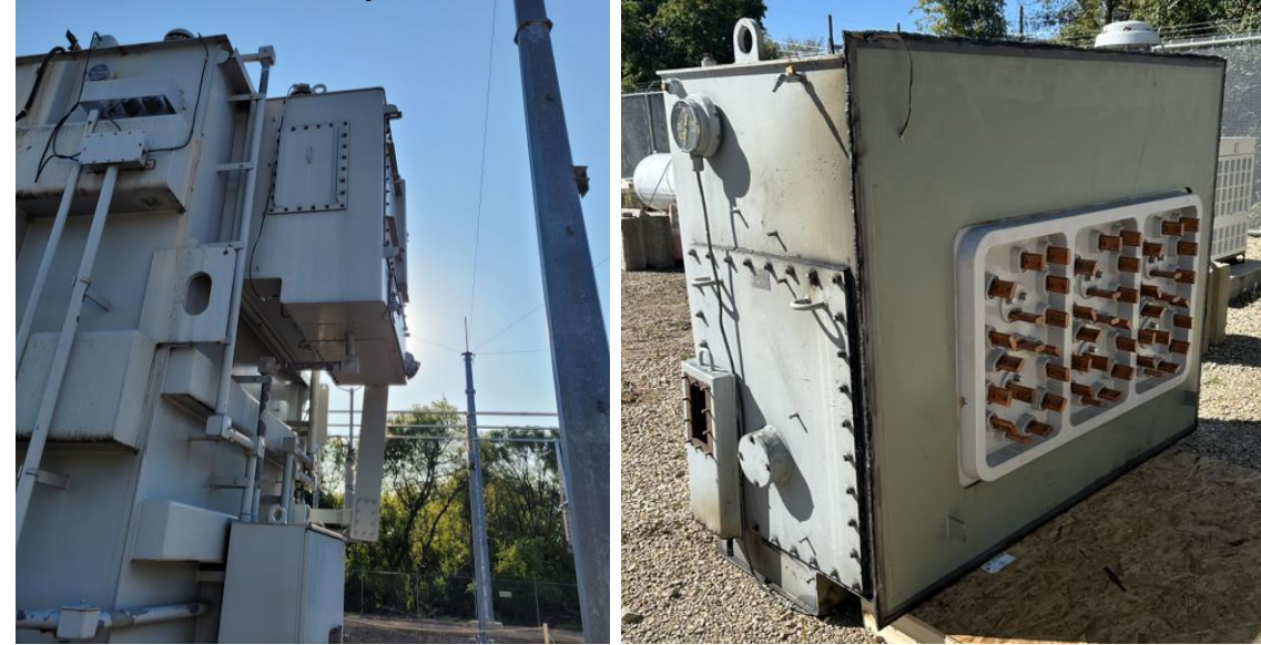
Before LTC Replacement
